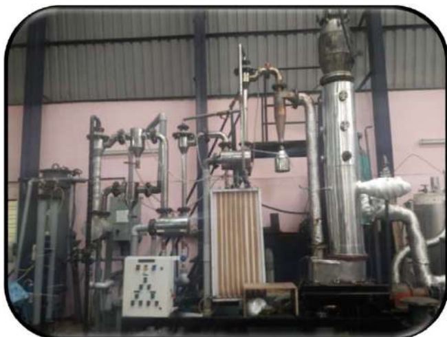
10 kW Biomass Gasification System
